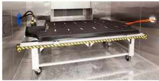
This is the Tesla battery inside the MILITARY-GRADE BLAST CHAMBER that it must be used in at the Tesla Factory because of the EXTREME EXPLOSION DANGER of the Tesla Battery
