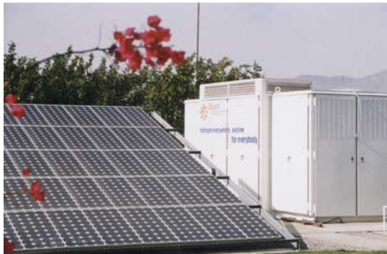
Figure 2 – The P3-1A Fleet Fuel Appliance at SunLine
