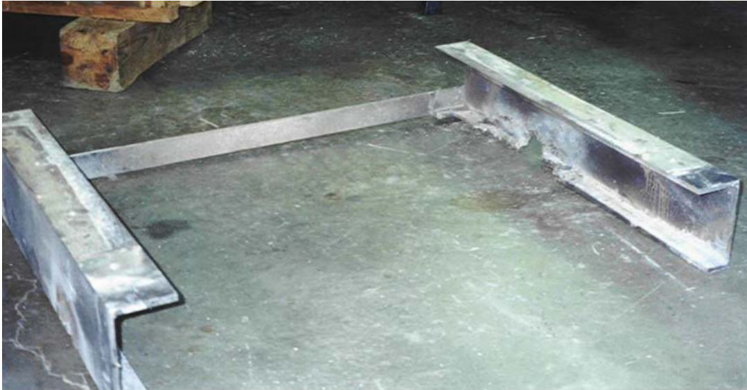
NJGenesis rear Battery Frame with Fire Damage
