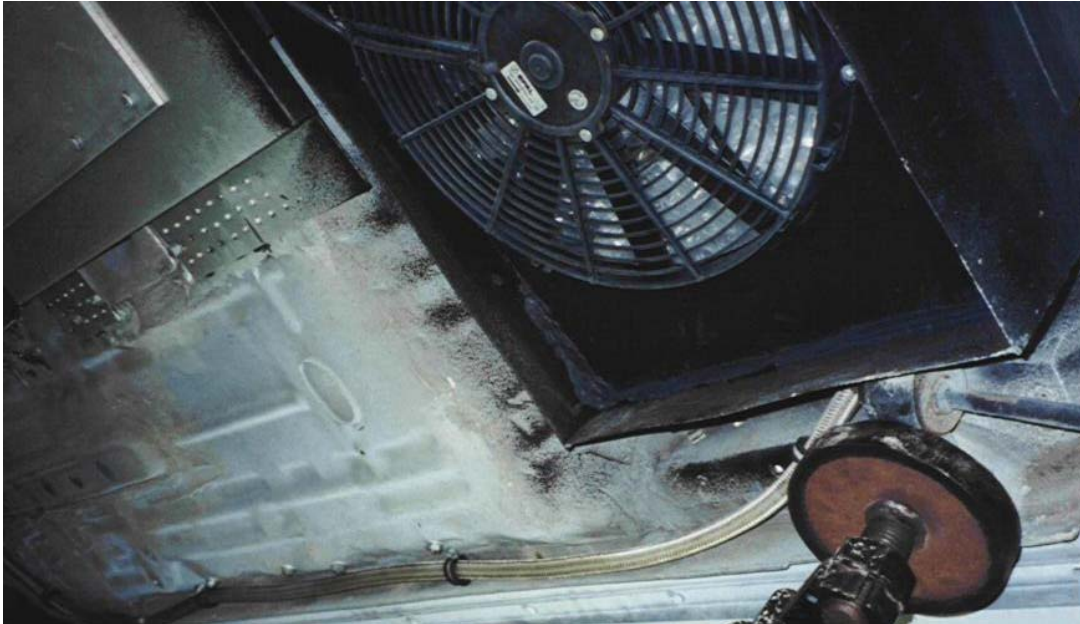
Figure 33 NJ Genesis underbody views - rear seat battery area cooling fan (1 of 2) installation.
