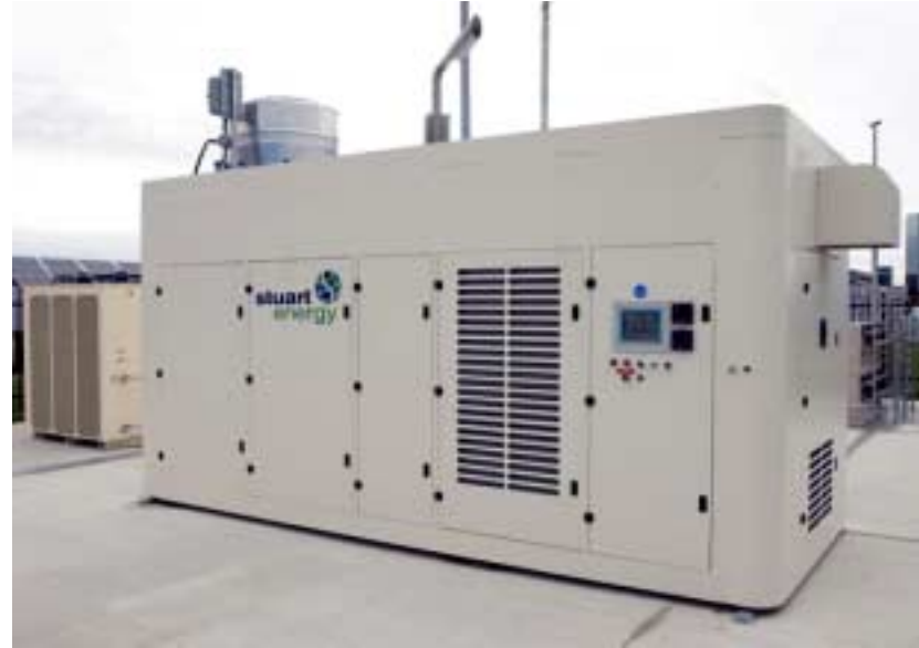
Electrolyzer (2.7kg/hr @ 5700psig)
