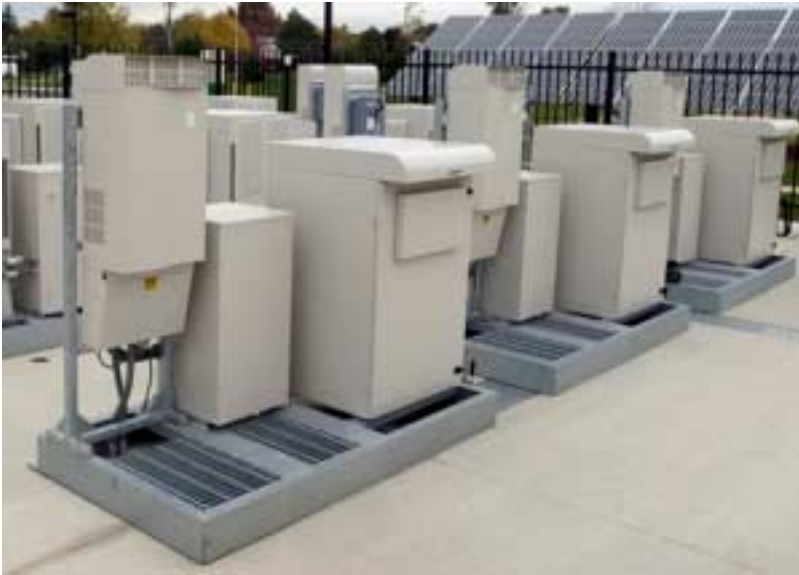
Fuel Cell Power System (50kW)
