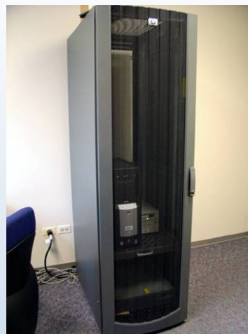
Server, workstation, tape backup and UPS
