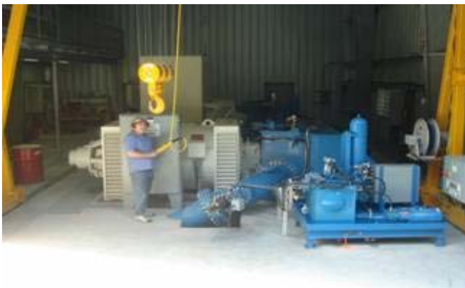
Generators in the Powerhouse at Brandywine Creek
