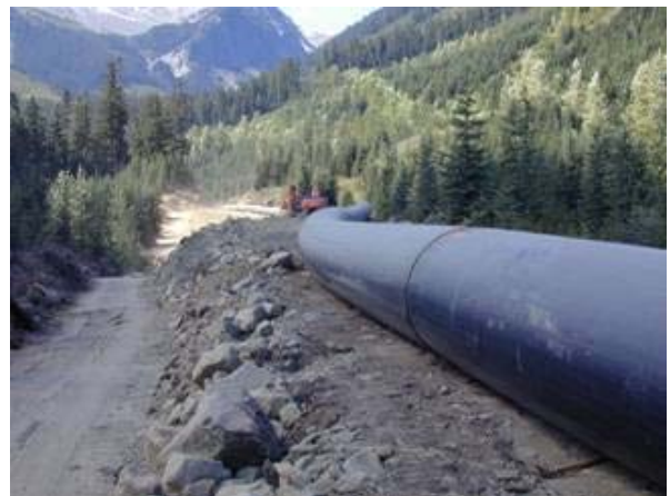
Penstock at Brandywine Creek
