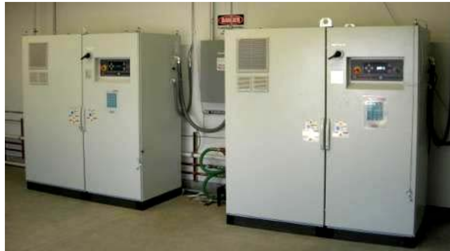
H6M Electrolyzers at Synthetic Energy
