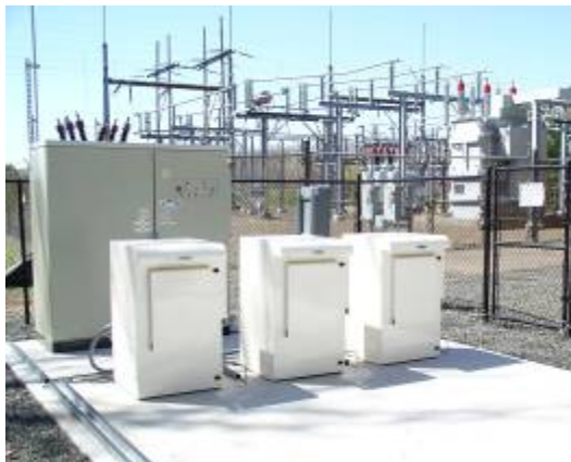
15 kW RFC backup power system, Wallingford, CT
