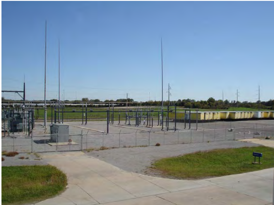
Figure 2.11. Proposed Site for the New Transformer
