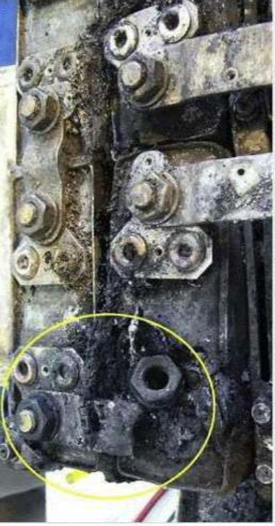
HERE IS THE BATTERY YOU COULD HAVE BEEN SITTING ON TOP OF IN A TESLA
